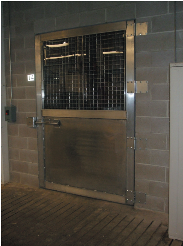
Figure 1.5 An isolation stall with its own ventilation system.
